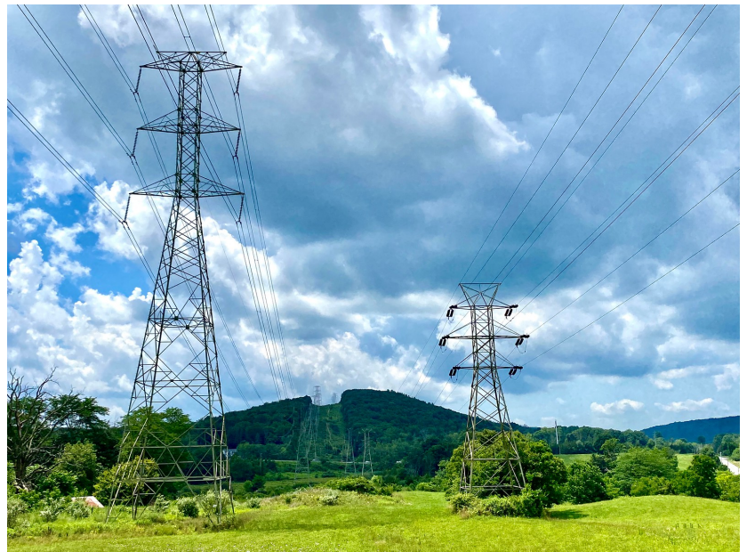
View of the transmission corridor with the larger structure holding the new Transco-owned 345 kV line.
